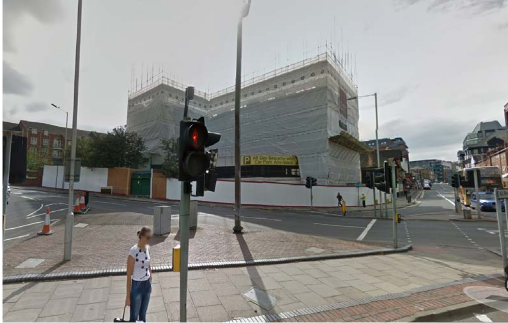
Photo of the former Kings Point building in September 2016, hoarded and undergoing demolition.
